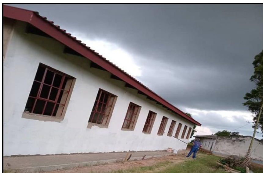
Picture 5: Ongoing rehabilitation at Lwandle RC Primary School under the AUC Project.
